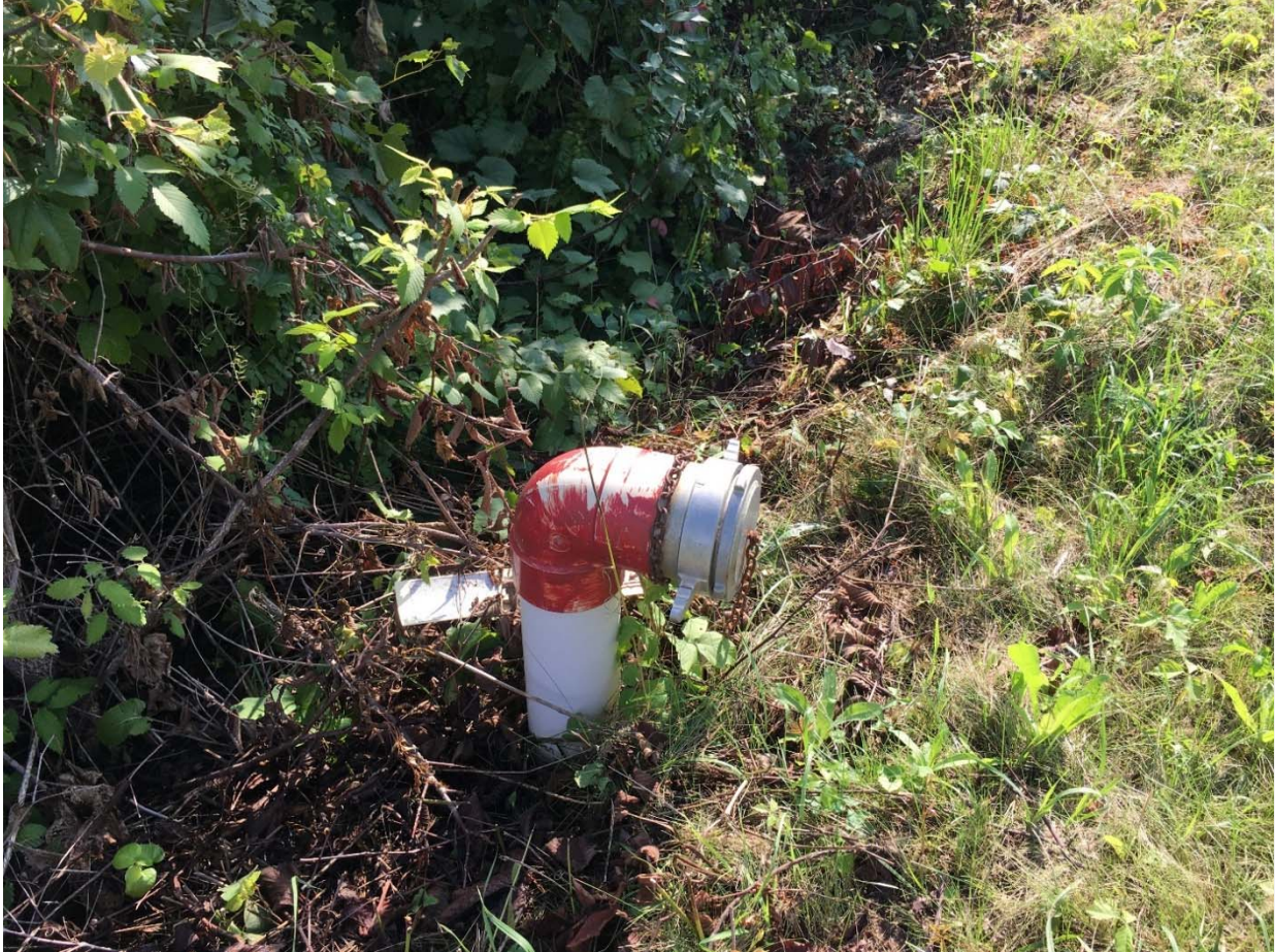
DRY HYDRANT LOCATED ALONG WEST UPSTREAM BANK
