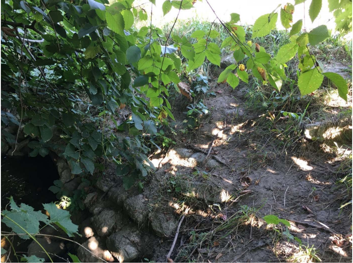
MINOR EROSION A DOWNSTREAM BANK
