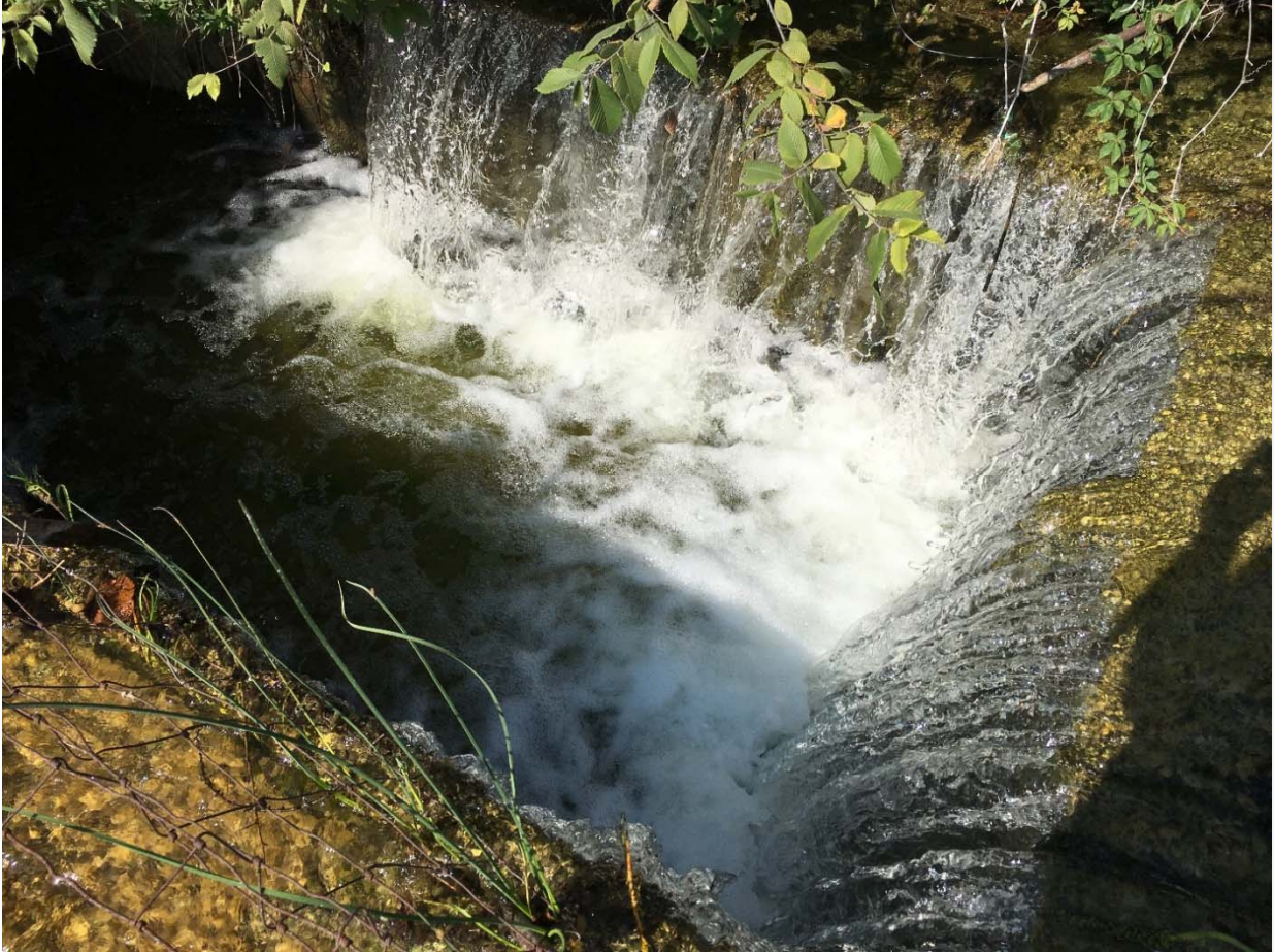
CLOSE UP OF OVERFLOW STRUCTURE – OUTLET PIPE TO LEFT; UPSTREAM CHANEL TO RIGHT
