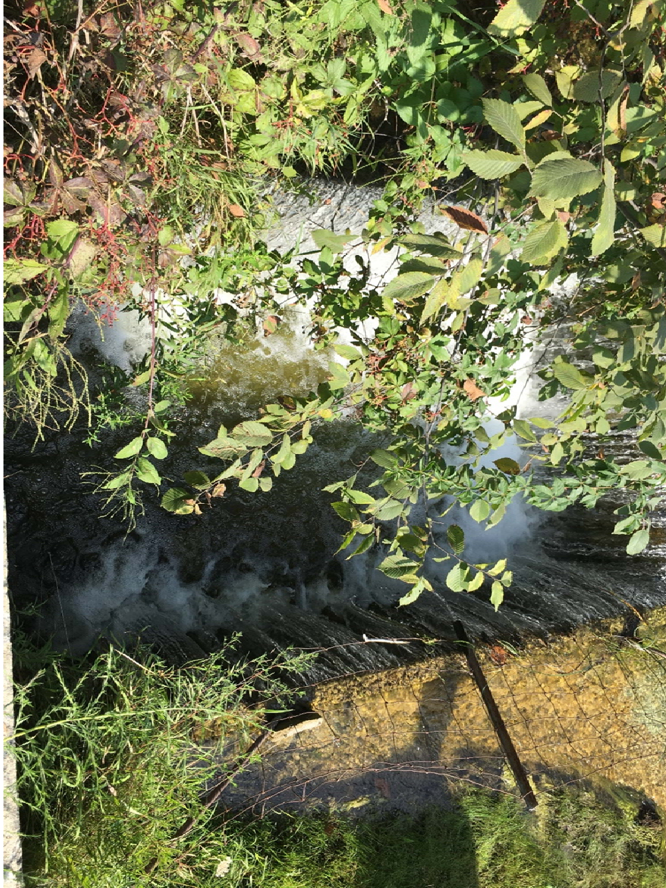
VIEW OF CONROL STRUCTURE - NOTE HEAVY VEGATATIVE GROWTH
