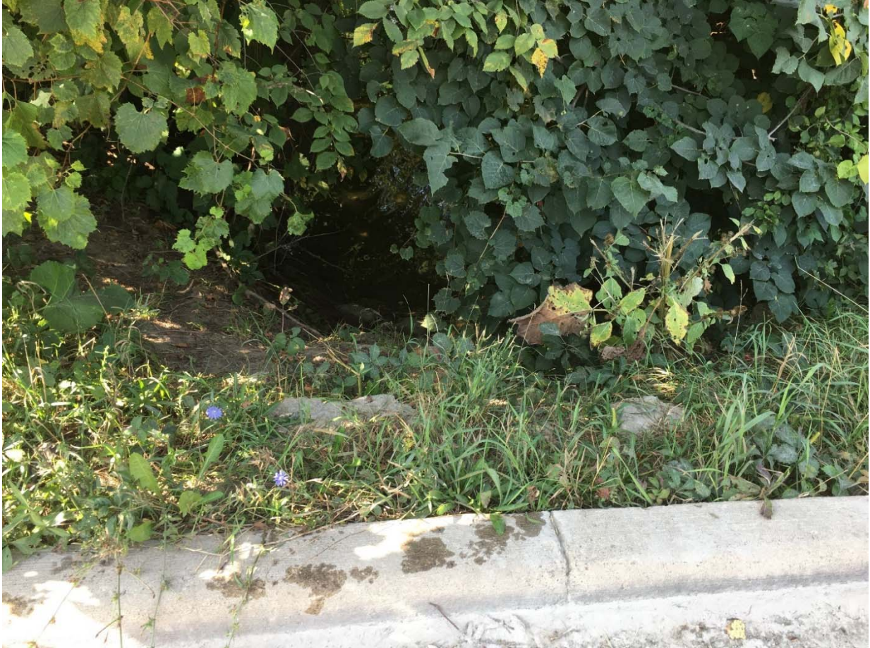
LOOKING SOUTH AT CONCRETE CURB SHOWING MINOR EROSION OVER OUTLET PIPE
