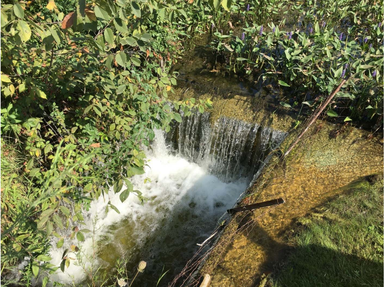
VIEW OF CONROL STRUCTURE – NOTE HEAVY WATER VEGETATION GROWTH
