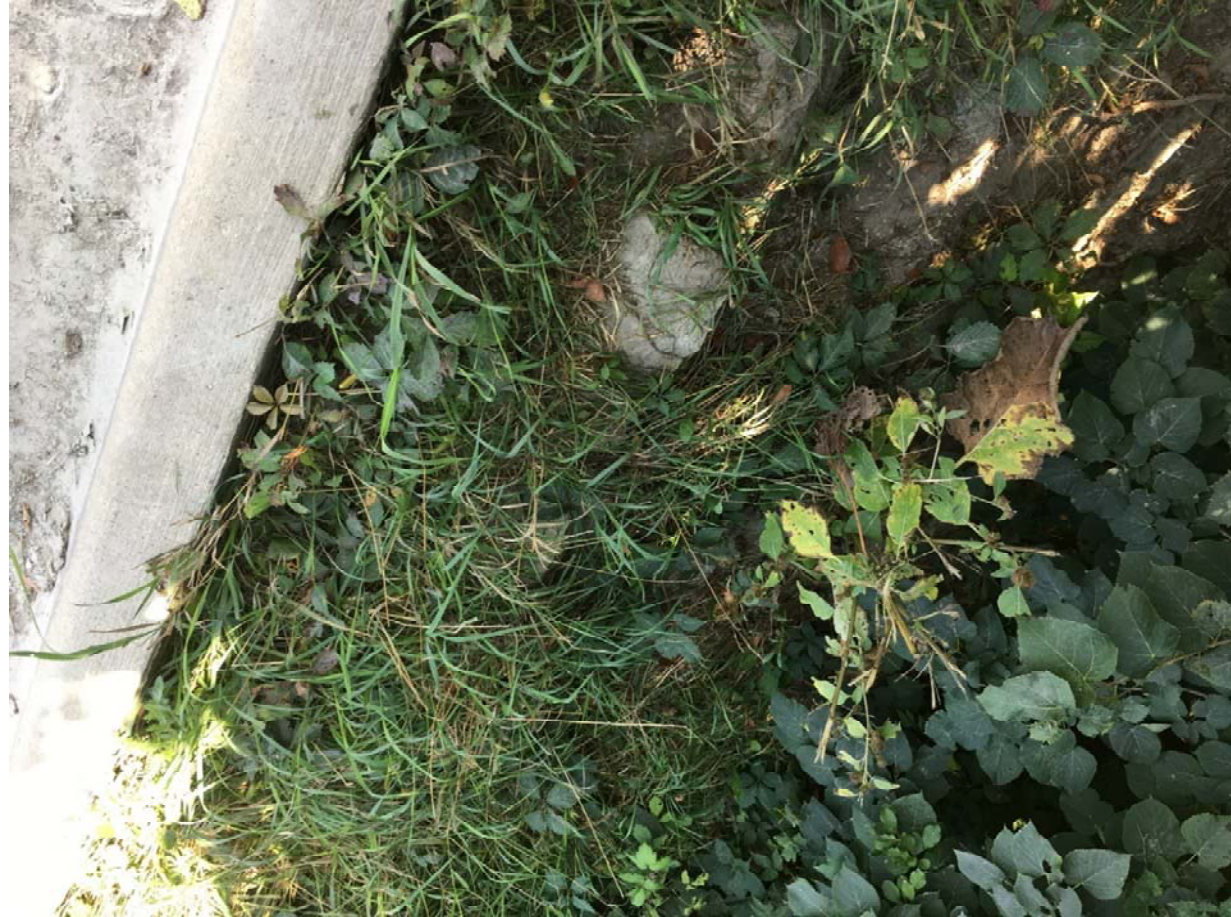
SETTELEMENT/EROSION BEHIND SOUTH ROADWAY CURB OVER OUTLET PIPE
