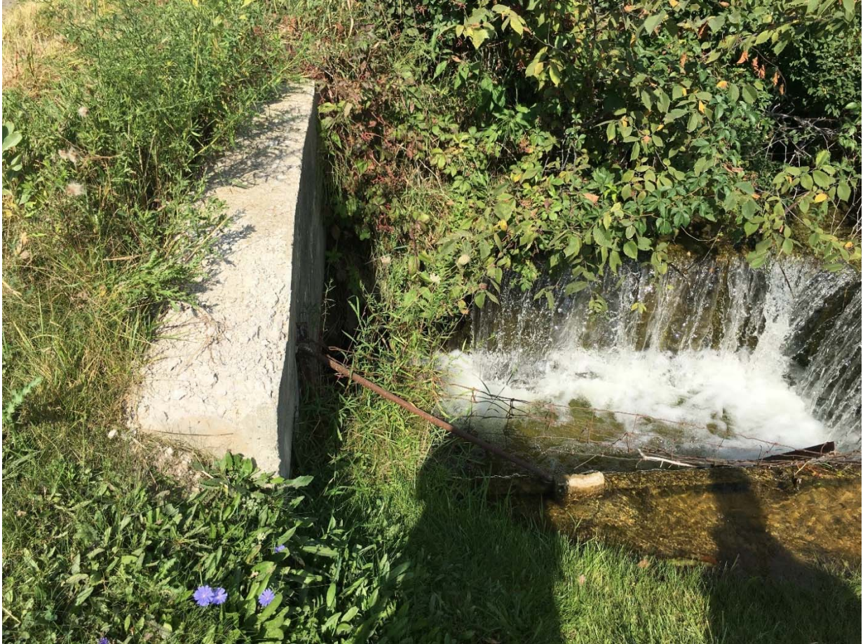
LOOKING WEST AT CONCRETE HEADWALL (LEFT) AND CONTROL STRUCTURE (RIGHT) NOTE HEADWALL SPALLING AND DELAMINATION
